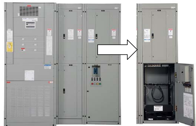
Before W.R. Controls
